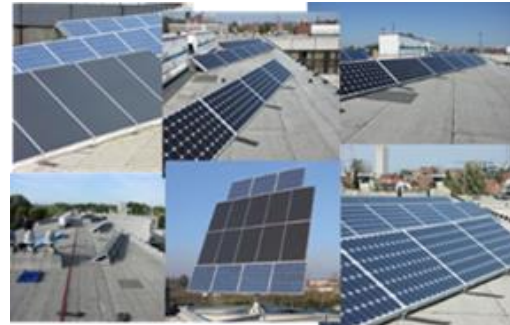
[PHOTO 2] : PV Test-field
