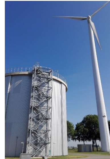
Breda (The Netherlands) digester \approx 8935\text{m}^3
