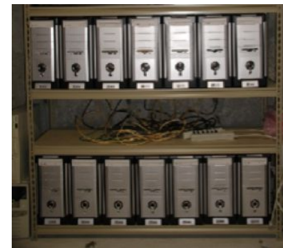
"Rack" with desktop PCs in a basement
